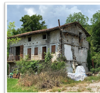
Mom's family home deemed "uninhabitable" from the earthquake
